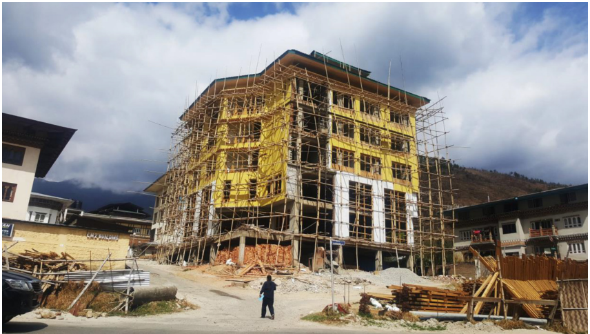
Plate 3: An almost complete 6-storey residential complex in Kawajangsa, Thimphu. The ground floor will be rented out as commercial space. The structure is RCC with brick walls and window frames are wood.
